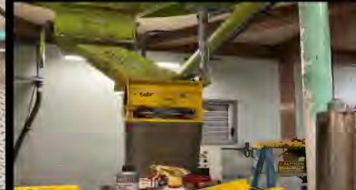
Rebuilt Lime Feeder
